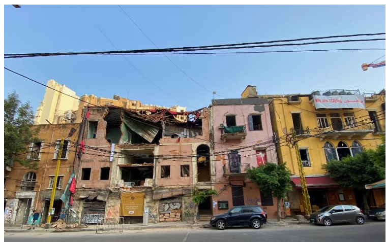
Above: damaged shelters from explosion in Mar Mikhael, Beirut – where ADRA Lebanon will provide cash-transfers
