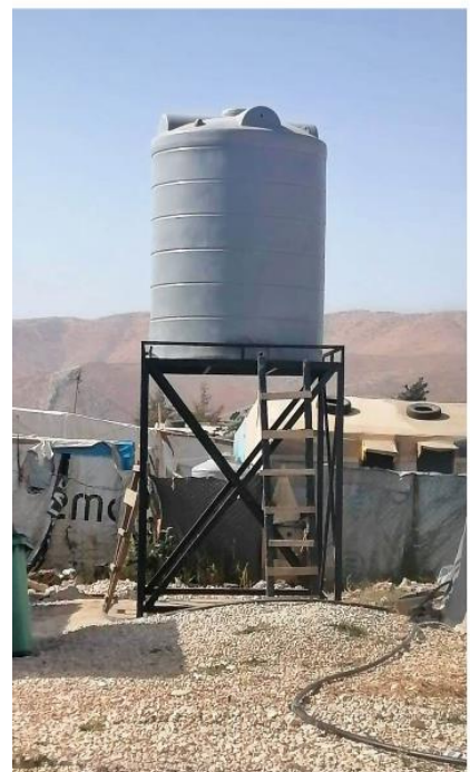
Photos - Top: 500-cubic meter water reservoir in Baalbek, Lebanon Bottom: elevated water tank in ITS - Bekaa, Lebanon
