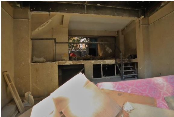
Above: damaged business which will receive ADRA's assistance
